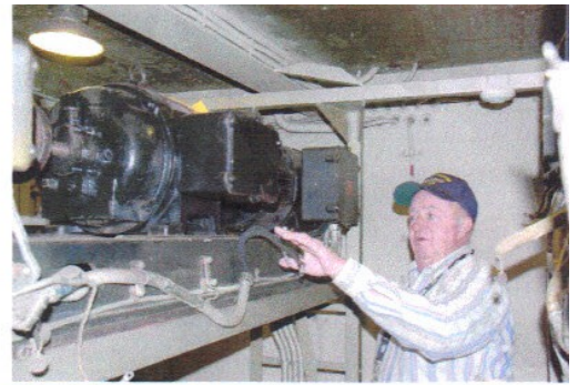
Norm showing the generators.
